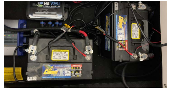
Hull Shield HS75 ultrasonic unit installed in the test boat.
