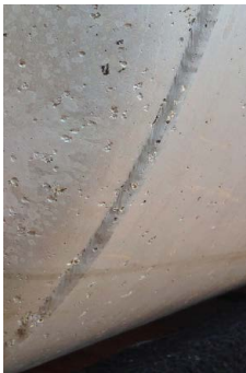
Above: Pitting caused by galvanic corrosion.
